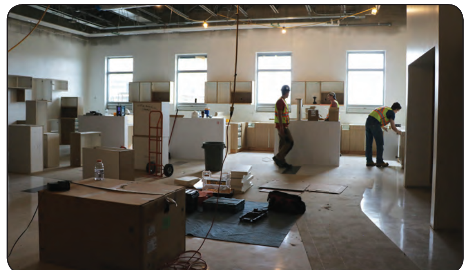
The school's spacious gym connects to two multi-purpose rooms. Right: Cabinets are already being installed in the home ec. room.
